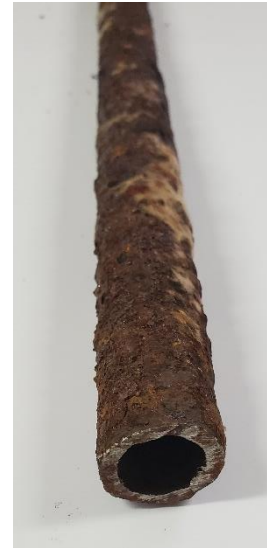
Figure 21: The corrosion looks alarming, but there is 90% sound metal in this riser pipe
